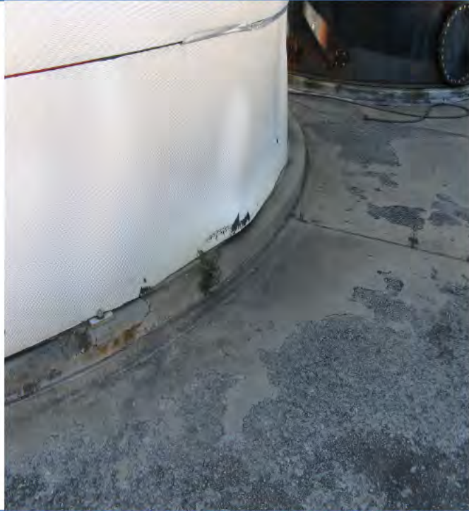
Photograph 1: Biodiesel Storage tank (bund area)
