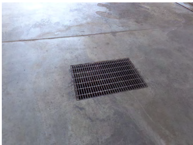
Photograph 5 – Blind sump in loading area
