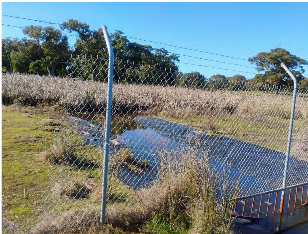
Photo 7: Lined drain connecting tailings pond to the water body
