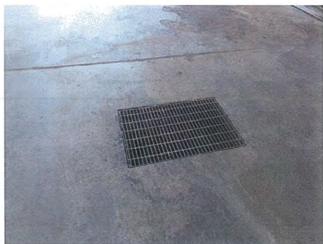
Photograph 5 – Blind sump in loading area
