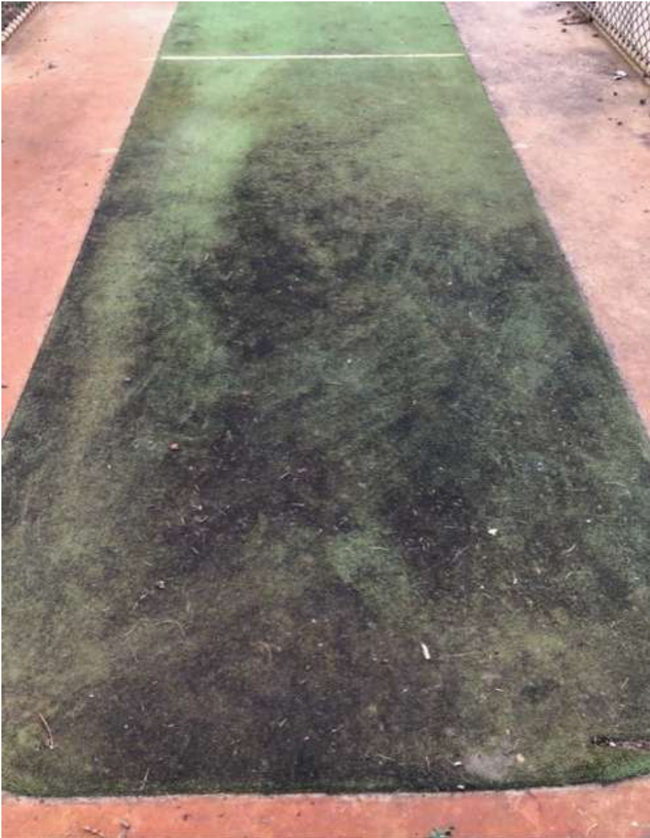
Net Carpet Damage Caused by Tree
