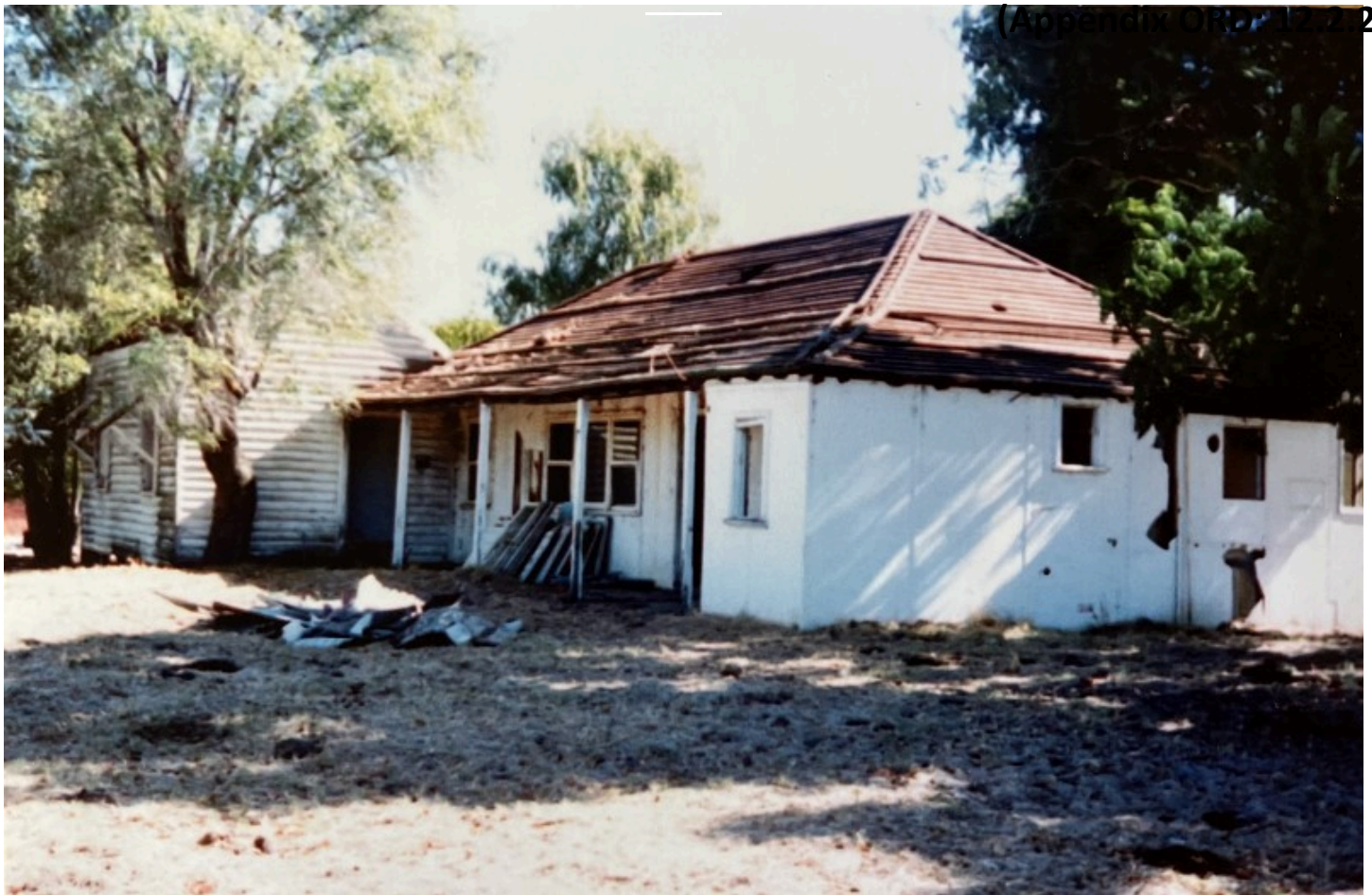
Killarney , the Garvey cottage unfortunately became unliveable due to heavy white-ant activity and was dismantled in 1988. The photograph shows the roof sheets removed to reveal the earlier timber shingle roof. The home represents a cottage typical of Dardanup in the 1850s. (Photograph; Jenny Golding – 1988)
