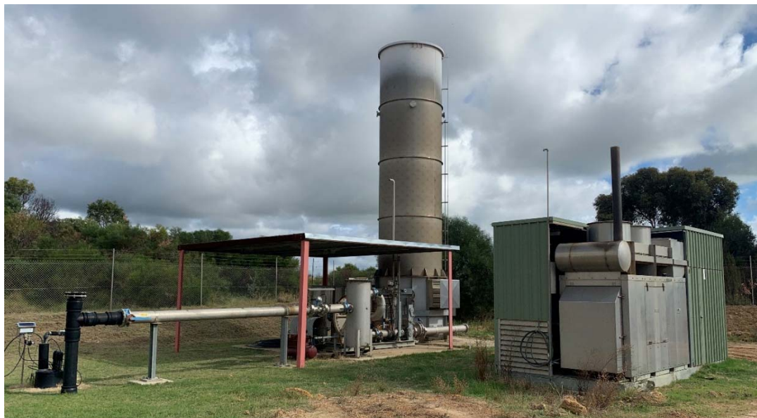
Figure 5 – Existing landfill gas flare and generator
