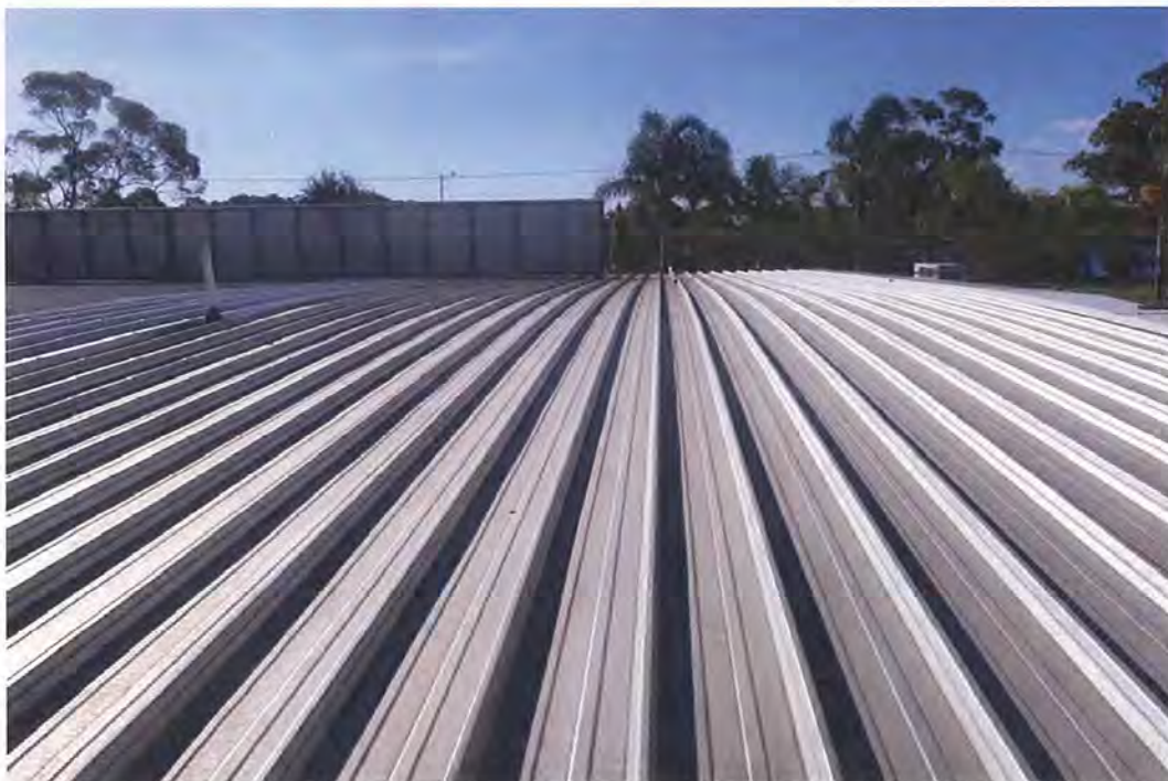
Sagging of roof planes puts the sheeting below its minimum recommended roof pitch.
