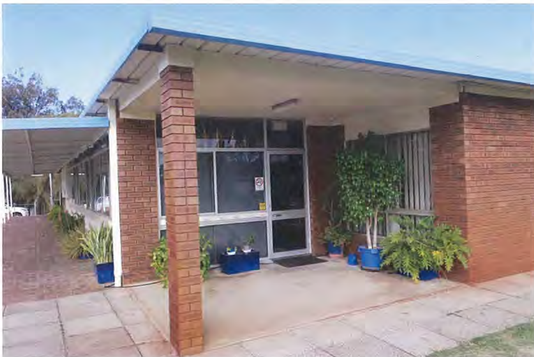
Corrosion in embedded steelwork is causing cracking of the masonry pier.
