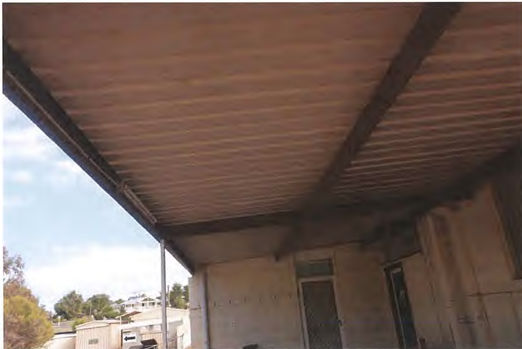
External structures with corrosion becoming evident and the sheeting being over span.
