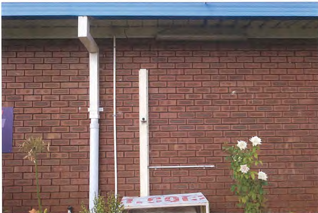
Evidence of settlement resulting in cracking of masonry elements.
