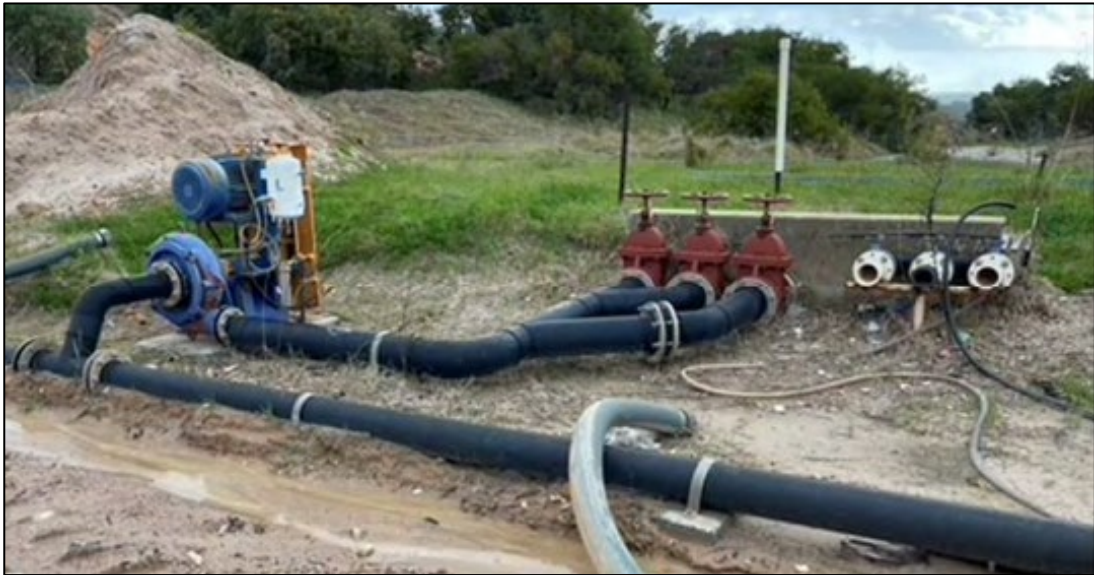
Existing tailings disposal point pump and infrastructure located adjacent to the existing workshop
