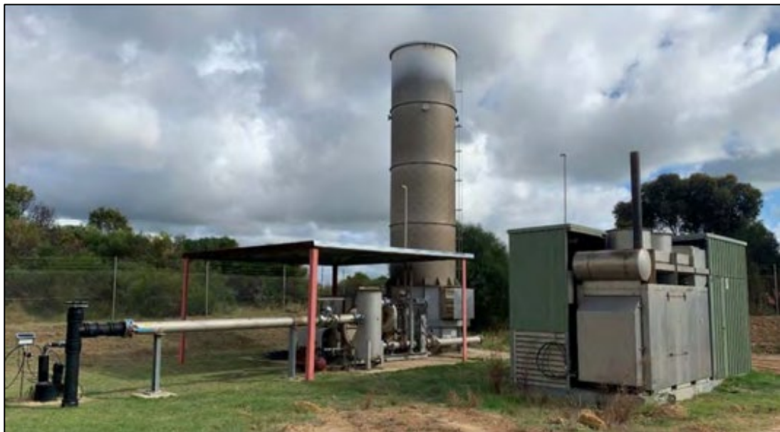
Existing landfill gas flare, generator, and air compressor unit
