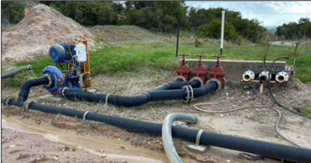
Existing tailings disposal point pump and infrastructure located adjacent to the existing workshop
