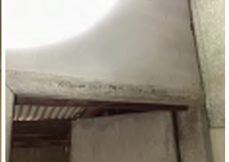
Showing examples of suspected asbestos
