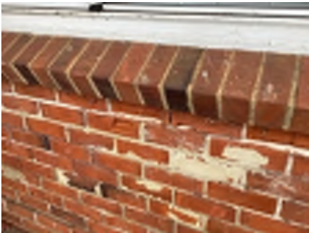
Cracking observed to parts of the external walls. Recommend a structural engineer be engaged to inspect and provide appropriate advice and recommendations to reduce the risk of further deterioration to the building.
