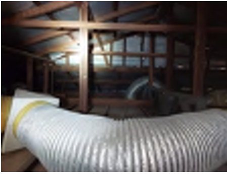
Showing example of insulation and AC duct to the ceiling space
