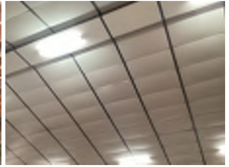
Showing examples of ceiling panels
