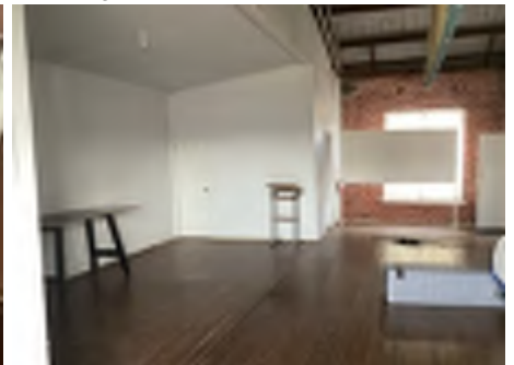
Showing example of uneven flooring
