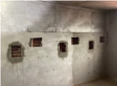
Showing examples of suspected asbestos
