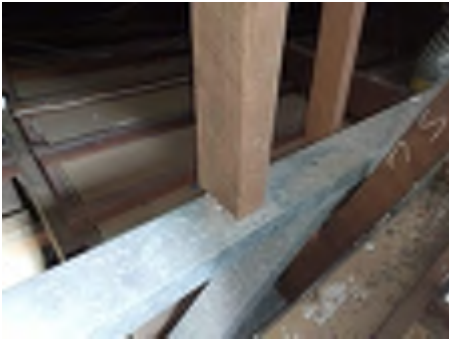
Angled bracing to beams to prevent rotation or movement is not observed to all areas. Recommend engaging a builder to repair to reduce the risk of movement and damage.
