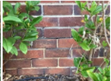
Cracking observed to parts of the external walls. Recommend a structural engineer be engaged to inspect and provide appropriate advice and recommendations to reduce the risk of further deterioration to the building.
