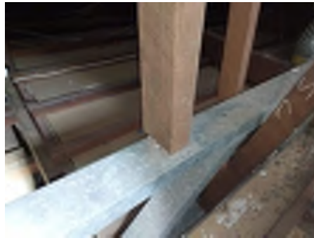
Timber struts bearing onto metal truss beams have no visual fasteners to the beams in some locations. Recommend engaging an engineer to investigate and a builder to repair to reduce the risk of movement and damage.
