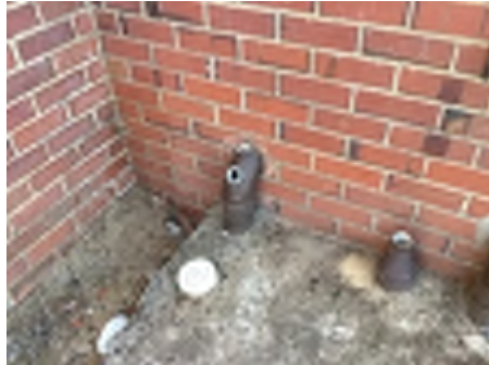
Showing plumbing pipe
