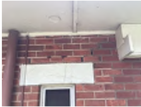
Cracking observed to parts of the external walls. Recommend a structural engineer be engaged to inspect and provide appropriate advice and recommendations to reduce the risk of further deterioration to the building.
