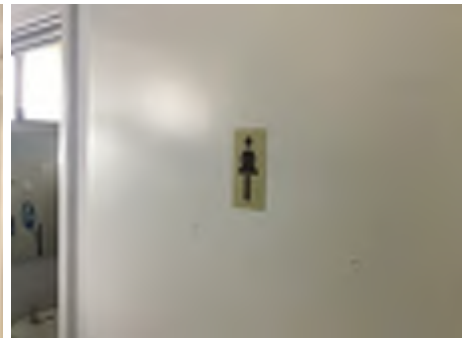
Cracking observed to parts of the internal walls. Recommend a structural engineer be engaged to inspect and provide appropriate advice and recommendations to reduce the risk of further deterioration to the building, To the rear kindergarten area.
