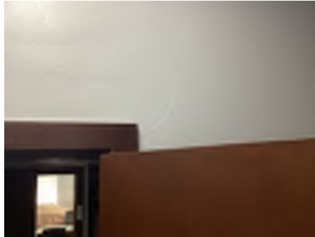
Cracking observed to parts of the internal walls. Recommend a structural engineer be engaged to inspect and provide appropriate advice and recommendations to reduce the risk of further deterioration to the building.
