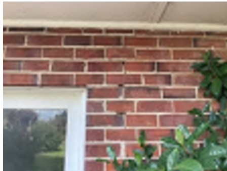
Cracking observed to parts of the external walls. Recommend a structural engineer be engaged to inspect and provide appropriate advice and recommendations to reduce the risk of further deterioration to the building.
