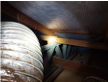
Timber struts bearing onto metal truss beams have no visual fasteners to the beams in some locations. Recommend engaging an engineer to investigate and a builder to repair to reduce the risk of movement and damage.
