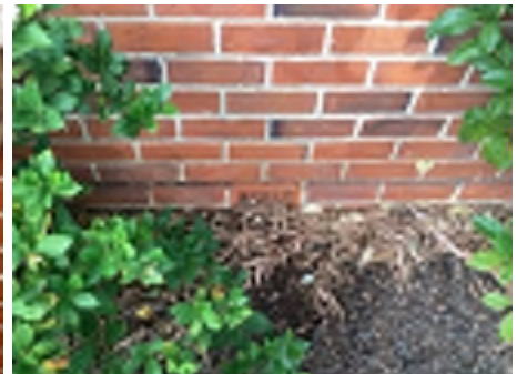
Cracking observed to parts of the external walls. Recommend a structural engineer be engaged to inspect and provide appropriate advice and recommendations to reduce the risk of further deterioration to the building.
