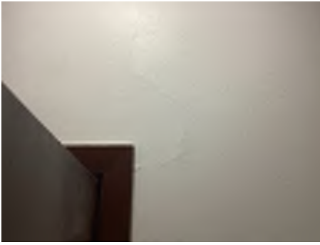
Cracking observed to parts of the internal walls. Recommend a structural engineer be engaged to inspect and provide appropriate advice and recommendations to reduce the risk of further deterioration to the building.
