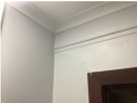
Cracking observed to parts of the internal walls. Recommend a structural engineer be engaged to inspect and provide appropriate advice and recommendations to reduce the risk of further deterioration to the building.
