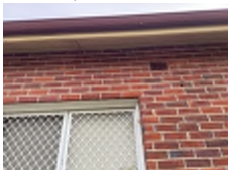
Cracking observed to parts of the external walls. Recommend a structural engineer be engaged to inspect and provide appropriate advice and recommendations to reduce the risk of further deterioration to the building.
