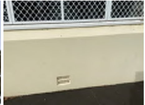
Cracking observed to parts of the external walls. Recommend a structural engineer be engaged to inspect and provide appropriate advice and recommendations to reduce the risk of further deterioration to the building.
