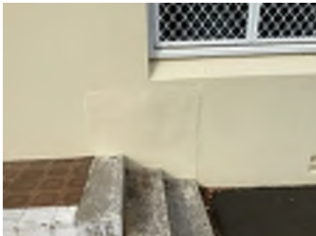
Cracking observed to parts of the external walls. Recommend a structural engineer be engaged to inspect and provide appropriate advice and recommendations to reduce the risk of further deterioration to the building.
