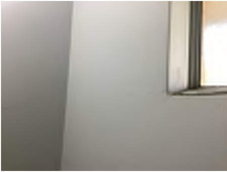
Cracking observed to parts of the internal walls. Recommend a structural engineer be engaged to inspect and provide appropriate advice and recommendations to reduce the risk of further deterioration to the building, To the rear kindergarten area.
