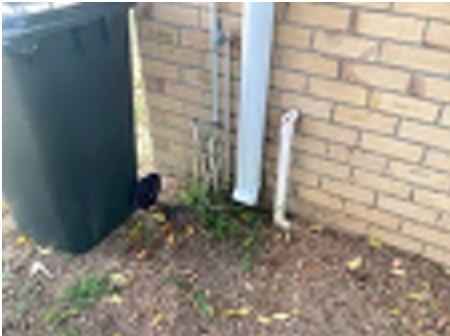
Showing earth wire
