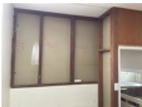
Showing examples of incomplete wall ovens
