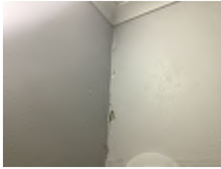
Cracking observed to parts of the internal walls. Recommend a structural engineer be engaged to inspect and provide appropriate advice and recommendations to reduce the risk of further deterioration to the building.
