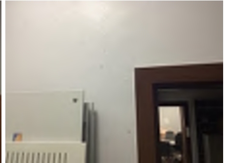
Cracking observed to parts of the internal walls. Recommend a structural engineer be engaged to inspect and provide appropriate advice and recommendations to reduce the risk of further deterioration to the building.
