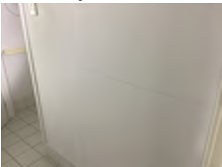
Cracking observed to parts of the internal walls. Recommend a structural engineer be engaged to inspect and provide appropriate advice and recommendations to reduce the risk of further deterioration to the building, To the rear kindergarten area.
