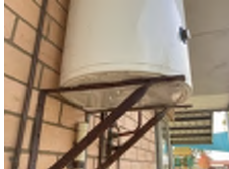
Showing hot water system
