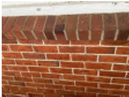
Cracking observed to parts of the external walls. Recommend a structural engineer be engaged to inspect and provide appropriate advice and recommendations to reduce the risk of further deterioration to the building.
