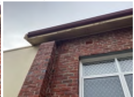
Cracking observed to parts of the external walls. Recommend a structural engineer be engaged to inspect and provide appropriate advice and recommendations to reduce the risk of further deterioration to the building.
