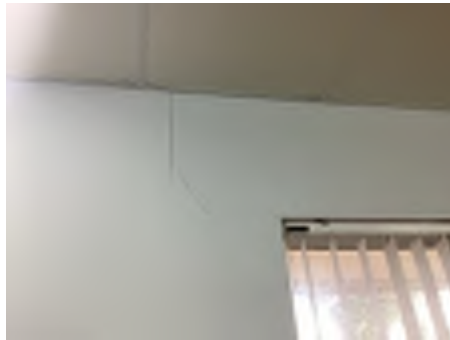
Cracking observed to parts of the internal walls. Recommend a structural engineer be engaged to inspect and provide appropriate advice and recommendations to reduce the risk of further deterioration to the building.
