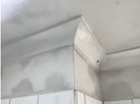
Showing examples of suspected mould
