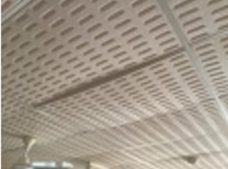
Showing examples of loose ceiling panels
