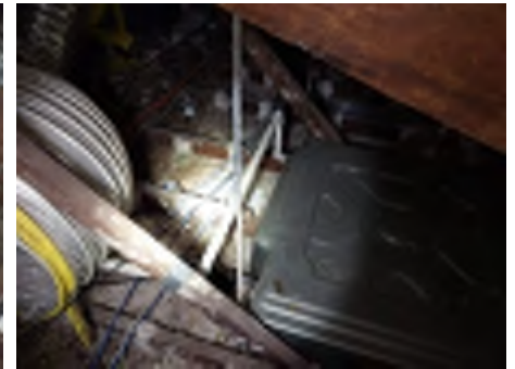
Ceiling timbers cut and not adequately reinforced around the AC position - recommend engaging a builder/ carpenter to repair to reduce the risk of damage.
