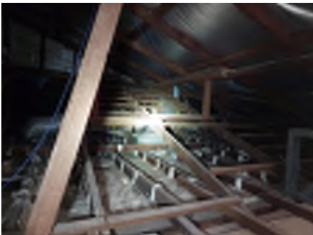
Some of the extension roofing members are propped onto the original roof structure with no additional support observed under the support load point. Recommend engaging an engineer to investigate and a builder to repair to reduce the risk of movement and damage.
