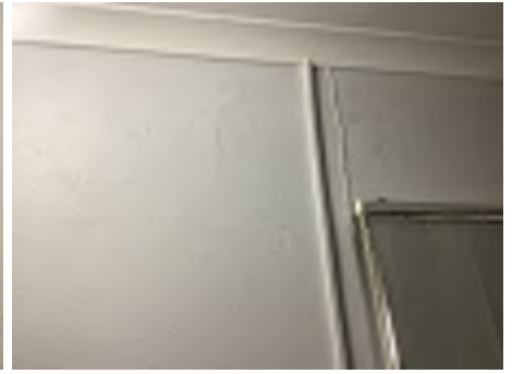
Cracking observed to parts of the internal walls. Recommend a structural engineer be engaged to inspect and provide appropriate advice and recommendations to reduce the risk of further deterioration to the building.
