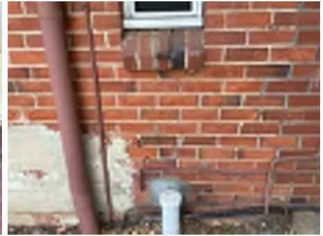
Cracking observed to parts of the external walls. Recommend a structural engineer be engaged to inspect and provide appropriate advice and recommendations to reduce the risk of further deterioration to the building.
