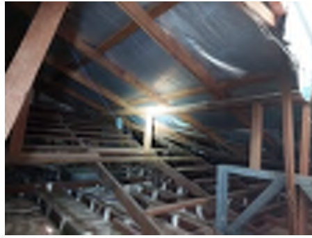
Spans to underpurlins are greater than typically allowed in several areas throughout the roof. Recommend engaging a builder to investigate and repair to reduce the risk of movement and damage.
