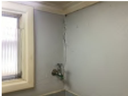
Cracking observed to parts of the internal walls. Recommend a structural engineer be engaged to inspect and provide appropriate advice and recommendations to reduce the risk of further deterioration to the building.
