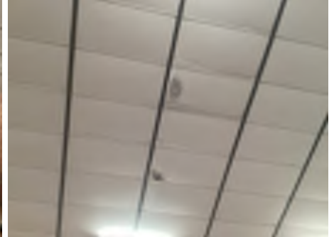
Showing examples of suspected mould
