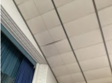
Showing examples of ceiling panels
