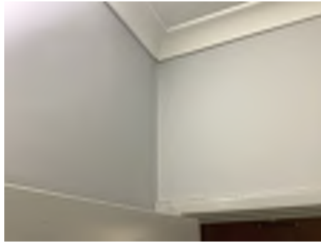
Cracking observed to parts of the internal walls. Recommend a structural engineer be engaged to inspect and provide appropriate advice and recommendations to reduce the risk of further deterioration to the building, To the rear kindergarten area.
