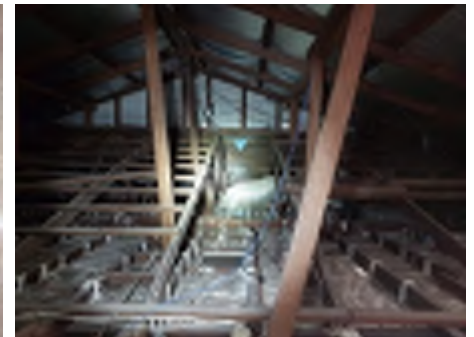
Some of the extension roofing members are propped onto the original roof structure with no additional support observed under the support load point. Recommend engaging an engineer to investigate and a builder to repair to reduce the risk of movement and damage.
