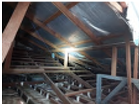
The roof cover appears to have been changed in the past to new roofing iron with modern fasteners. No provision to upgrade supporting timbers and tie downs to the roof to the requirements of the approximate date of the changed roof cover are observed. Recommend engaging an engineer to assess and a builder to install additional timbers, tie downs and strapping or obtaining a signed engineering detail for the roof change as constructed.
