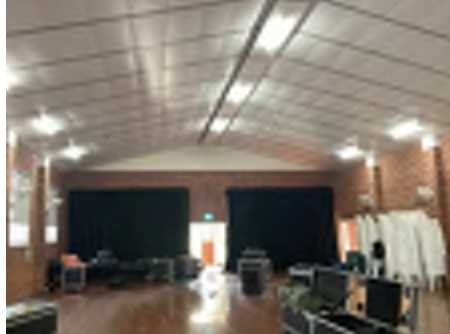
Showing examples of ceiling panels
