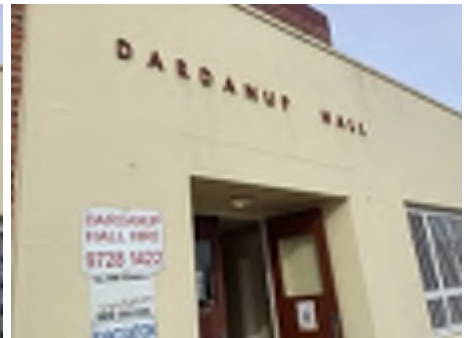
Cracking observed to parts of the external walls. Recommend a structural engineer be engaged to inspect and provide appropriate advice and recommendations to reduce the risk of further deterioration to the building.
