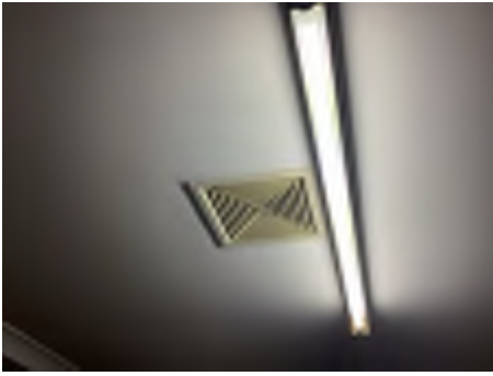
Showing example of ceiling vents
