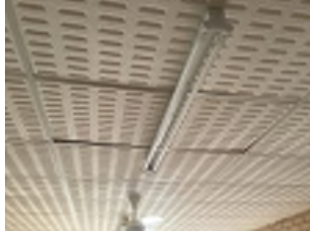
Showing examples of loose ceiling panels
