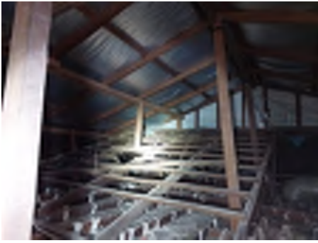
Some of the extension roofing members are propped onto the original roof structure with no additional support observed under the support load point. Recommend engaging an engineer to investigate and a builder to repair to reduce the risk of movement and damage.
