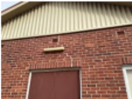
Cracking observed to parts of the external walls. Recommend a structural engineer be engaged to inspect and provide appropriate advice and recommendations to reduce the risk of further deterioration to the building.
