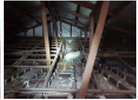
Spans to underpurlins are greater than typically allowed in several areas throughout the roof. Recommend engaging a builder to investigate and repair to reduce the risk of movement and damage.
