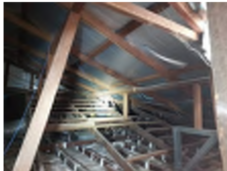
Some of the extension roofing members are propped onto the original roof structure with no additional support observed under the support load point. Recommend engaging an engineer to investigate and a builder to repair to reduce the risk of movement and damage.
