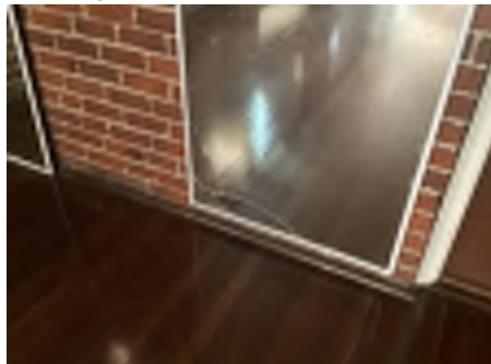
Showing cracked mirror
