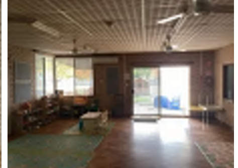
Showing examples of loose ceiling panels
