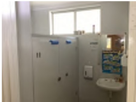
Cracking observed to parts of the internal walls. Recommend a structural engineer be engaged to inspect and provide appropriate advice and recommendations to reduce the risk of further deterioration to the building, To the rear kindergarten area.
