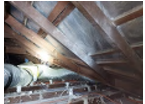
The roof cover appears to have been changed in the past to new roofing iron with modern fasteners. No provision to upgrade supporting timbers and tie downs to the roof to the requirements of the approximate date of the changed roof cover are observed. Recommend engaging an engineer to assess and a builder to install additional timbers, tie downs and strapping or obtaining a signed engineering detail for the roof change as constructed.
