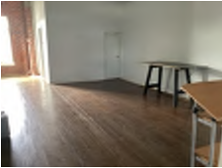
Showing example of uneven flooring
