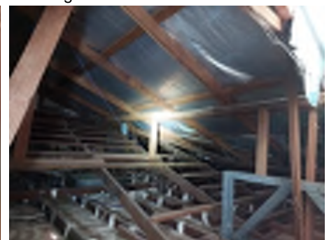
Showing example of insulation and AC duct to the ceiling space
