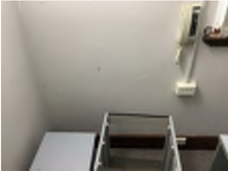
Cracking observed to parts of the internal walls. Recommend a structural engineer be engaged to inspect and provide appropriate advice and recommendations to reduce the risk of further deterioration to the building.
