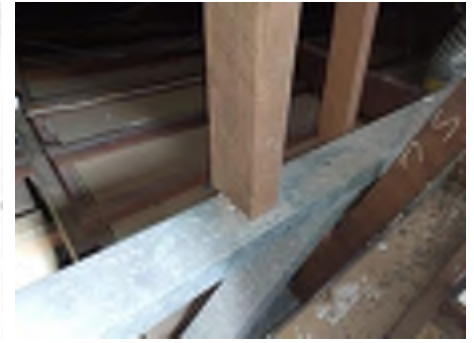
Timber struts bearing onto metal truss beams have no visual fasteners to the beams in some locations. Recommend engaging an engineer to investigate and a builder to repair to reduce the risk of movement and damage.
