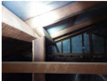
Spans to underpurlins are greater than typically allowed in several areas throughout the roof. Recommend engaging a builder to investigate and repair to reduce the risk of movement and damage.
