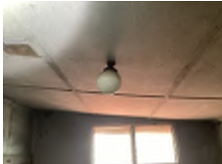
Showing examples of suspected asbestos
