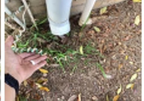
Showing earth wire
