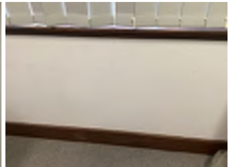
Cracking observed to parts of the internal walls. Recommend a structural engineer be engaged to inspect and provide appropriate advice and recommendations to reduce the risk of further deterioration to the building.
