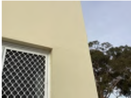
Cracking observed to parts of the external walls. Recommend a structural engineer be engaged to inspect and provide appropriate advice and recommendations to reduce the risk of further deterioration to the building.
