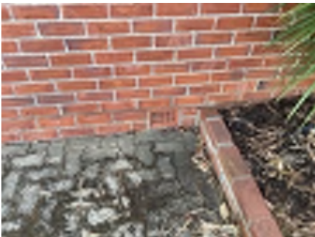
Cracking observed to parts of the external walls. Recommend a structural engineer be engaged to inspect and provide appropriate advice and recommendations to reduce the risk of further deterioration to the building.
