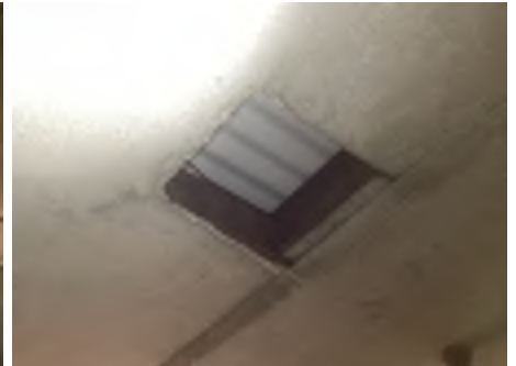
Showing examples of suspected asbestos
