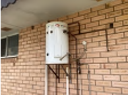
Showing hot water system
