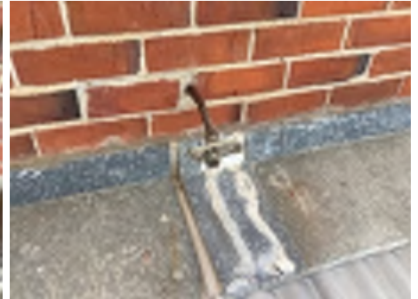
Showing examples of exposed wires
