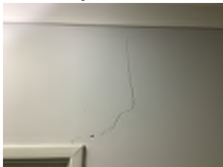
Cracking observed to parts of the internal walls. Recommend a structural engineer be engaged to inspect and provide appropriate advice and recommendations to reduce the risk of further deterioration to the building, To the rear kindergarten area.
