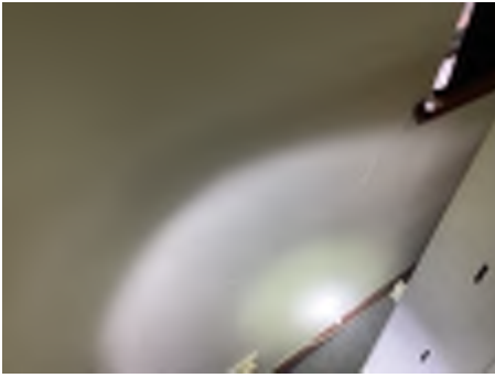
Cracking observed to parts of the internal walls. Recommend a structural engineer be engaged to inspect and provide appropriate advice and recommendations to reduce the risk of further deterioration to the building.
