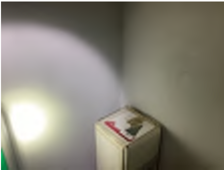
Cracking observed to parts of the internal walls. Recommend a structural engineer be engaged to inspect and provide appropriate advice and recommendations to reduce the risk of further deterioration to the building.
