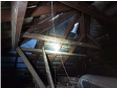
Spans to underpurlins are greater than typically allowed in several areas throughout the roof. Recommend engaging a builder to investigate and repair to reduce the risk of movement and damage.
