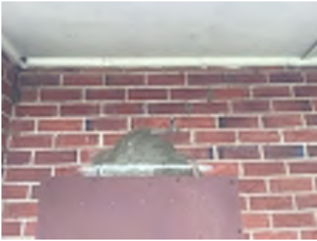
Cracking observed to parts of the external walls. Recommend a structural engineer be engaged to inspect and provide appropriate advice and recommendations to reduce the risk of further deterioration to the building.
