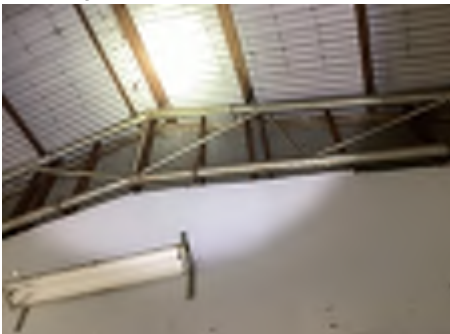
Showing examples of suspected asbestos
