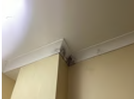
Showing examples of suspected mould
