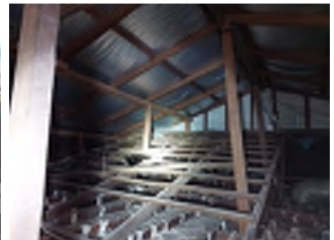
The roof cover appears to have been changed in the past to new roofing iron with modern fasteners. No provision to upgrade supporting timbers and tie downs to the roof to the requirements of the approximate date of the changed roof cover are observed. Recommend engaging an engineer to assess and a builder to install additional timbers, tie downs and strapping or obtaining a signed engineering detail for the roof change as constructed.
