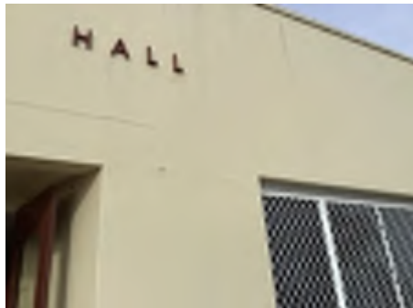
Cracking observed to parts of the external walls. Recommend a structural engineer be engaged to inspect and provide appropriate advice and recommendations to reduce the risk of further deterioration to the building.
