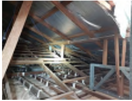
Timber struts bearing onto metal truss beams have no visual fasteners to the beams in some locations. Recommend engaging an engineer to investigate and a builder to repair to reduce the risk of movement and damage.
