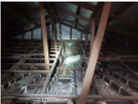
The roof cover appears to have been changed in the past to new roofing iron with modern fasteners. No provision to upgrade supporting timbers and tie downs to the roof to the requirements of the approximate date of the changed roof cover are observed. Recommend engaging an engineer to assess and a builder to install additional timbers, tie downs and strapping or obtaining a signed engineering detail for the roof change as constructed.
