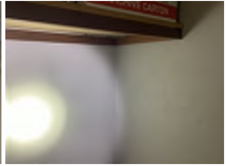
Cracking observed to parts of the internal walls. Recommend a structural engineer be engaged to inspect and provide appropriate advice and recommendations to reduce the risk of further deterioration to the building.
