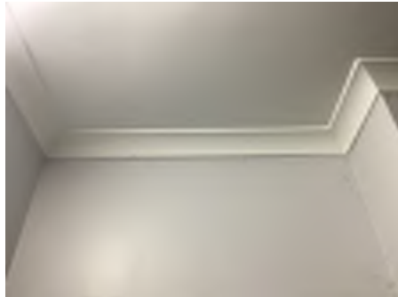
Cracking observed to parts of the internal walls. Recommend a structural engineer be engaged to inspect and provide appropriate advice and recommendations to reduce the risk of further deterioration to the building.
