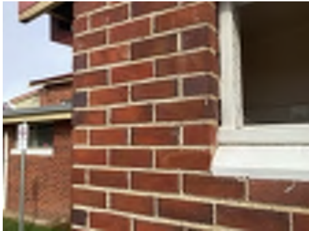
Cracking observed to parts of the external walls. Recommend a structural engineer be engaged to inspect and provide appropriate advice and recommendations to reduce the risk of further deterioration to the building.
