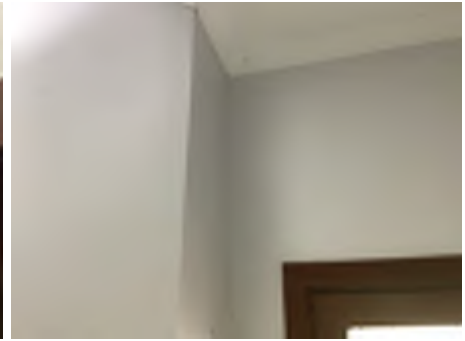
Cracking observed to parts of the internal walls. Recommend a structural engineer be engaged to inspect and provide appropriate advice and recommendations to reduce the risk of further deterioration to the building.
