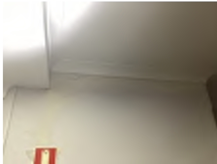
Cracking observed to parts of the internal walls. Recommend a structural engineer be engaged to inspect and provide appropriate advice and recommendations to reduce the risk of further deterioration to the building.
