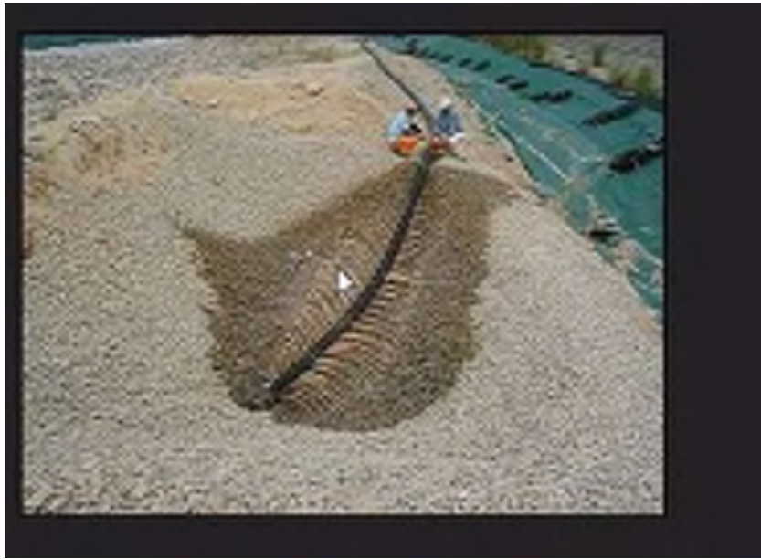
Operating UK Leachate Reticulation System showing the spray pattern.
