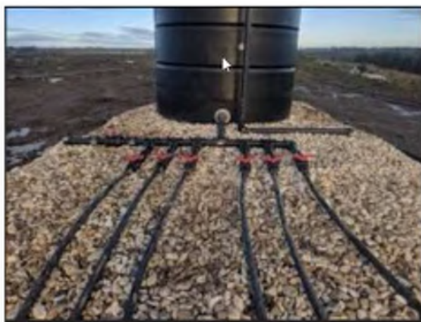
Image 1 – Leachate Reticulation System in operation in the UK. Image provided by Cleanaway.
