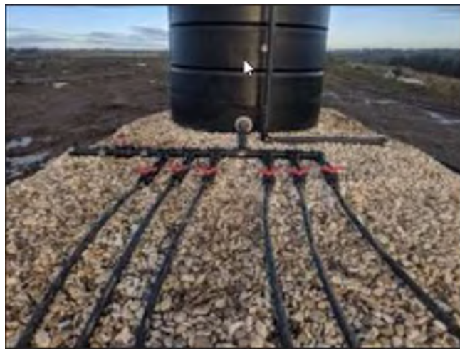
Operating UK Leachate Reticulation System
