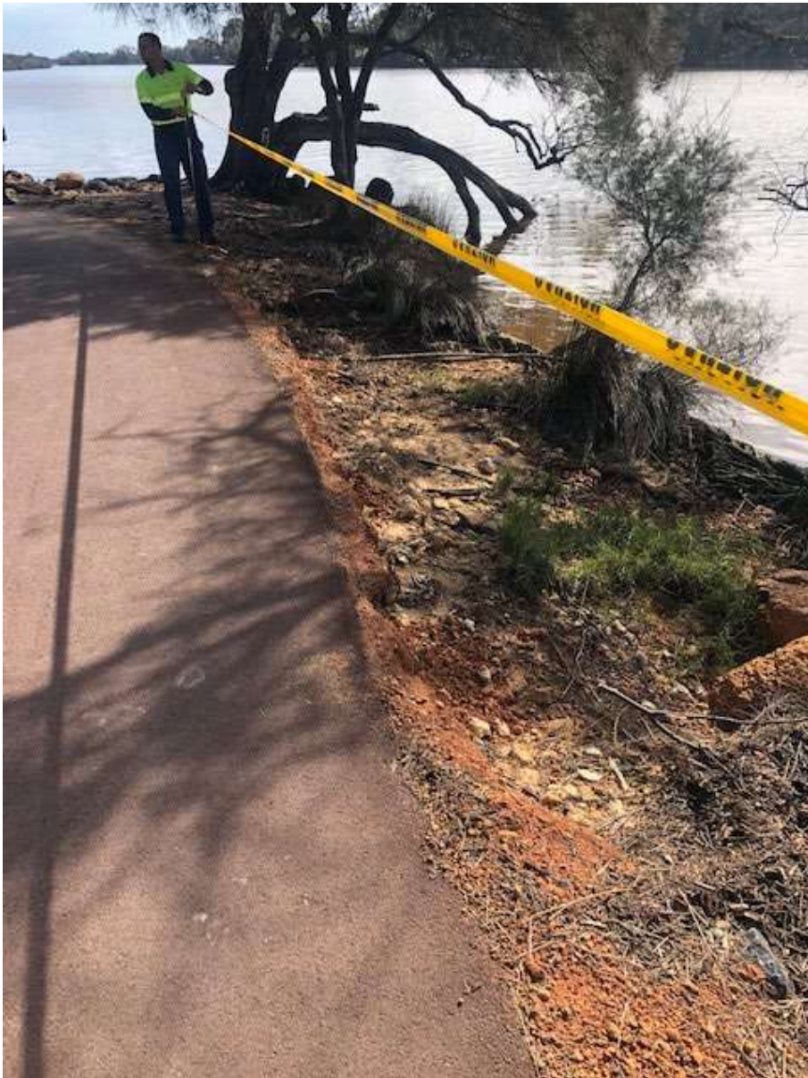
Storm Damage from August 2022 within the Shire of Dardanup
