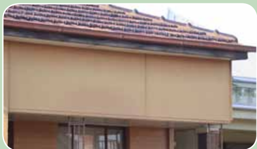
Asbestos cement sheeting in eaves
