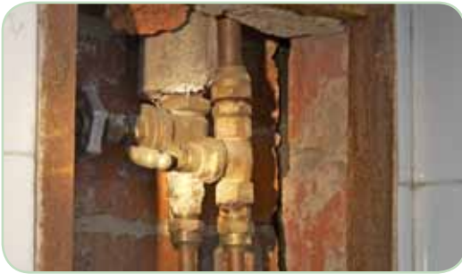
Friable asbestos lagging on pipes
